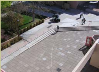
Water Leakage Investigation Centennial Library, Univ. of New Mexico Albuquerque, New Mexico
